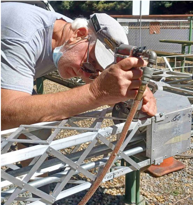
Following weeks of effort, John Davis drives the final rivets to repair the signal bridge that had been damaged in a storm last winter.
